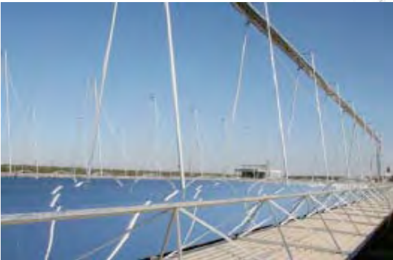
Kimberlina 5 MW Bakersfield, California
